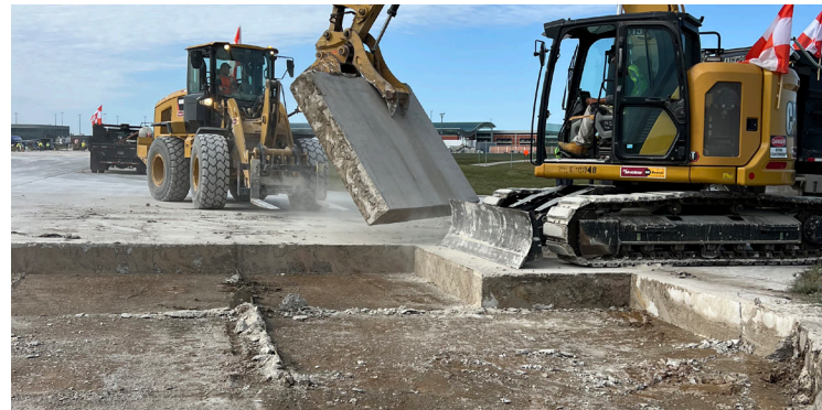
Pavement repairs at the Gerald R. Ford International Airport in Grand Rapids, Michigan, capturing pavement demolitions
